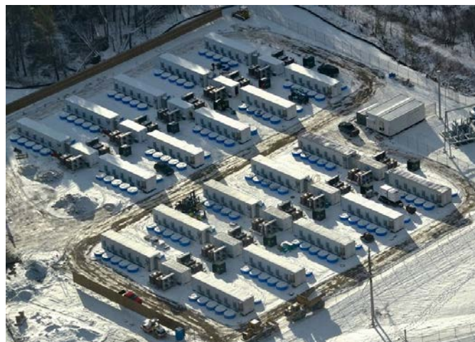
Imagen 22 Beacon Power's Stephentown Flywheel Energy Storage Plant
