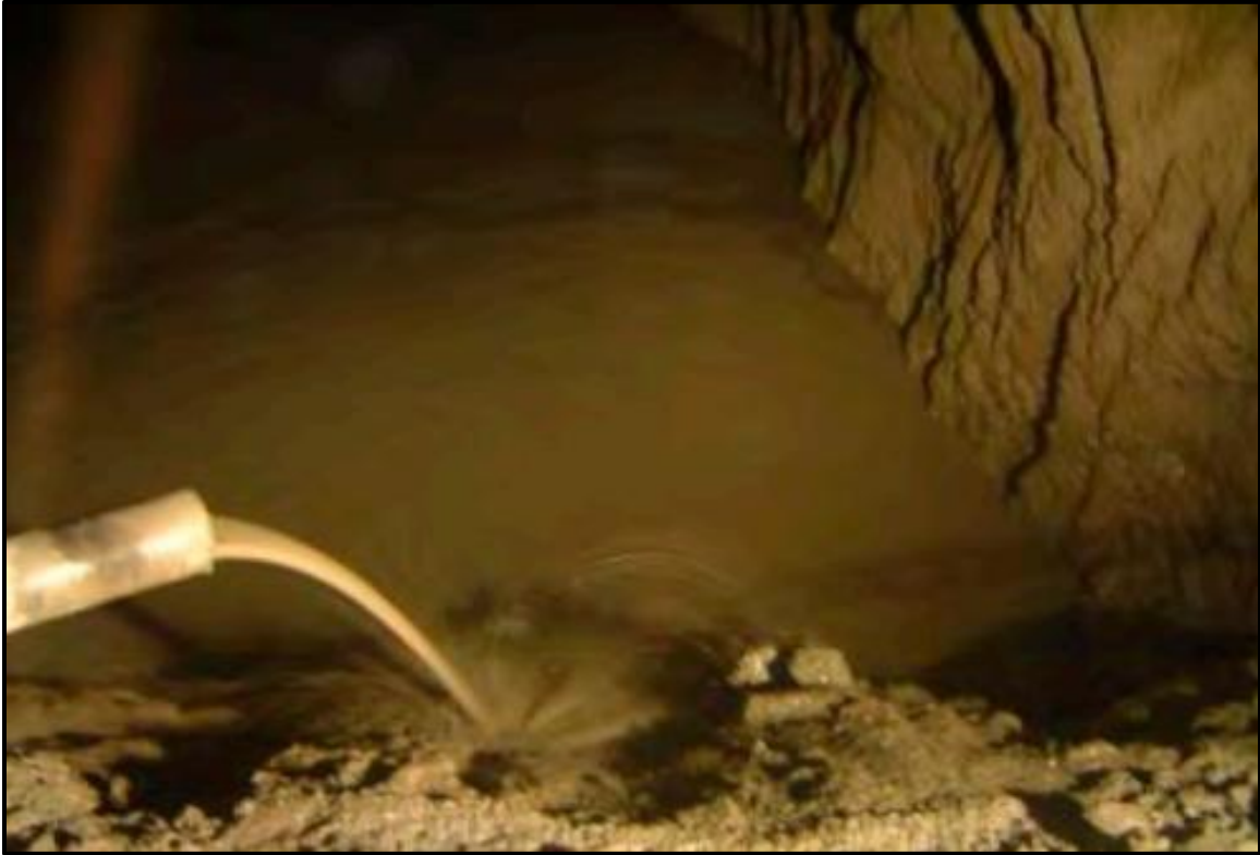
Figura 4. 2. Relleno con jales de obra subterránea en mina de Perú. Fuente: Experiences of Underground Mine Backfilling Using Mine Tailings Developed in the Andean Region of Peru: A Green Mining Solution to Reduce Socio-Environmental Impacts (Cacciattolo & Marinovic, 2023).
