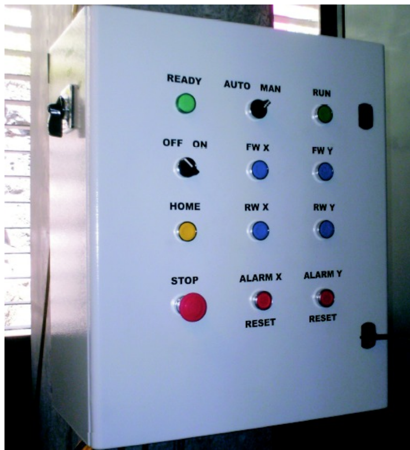
Figura 7.2: Panel de control
