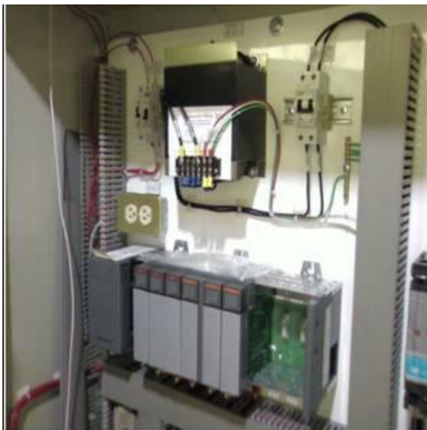
Figura 4.171. Tablero de control “PC” con interruptor general y PLC de control principal (Baselis, 2010)
