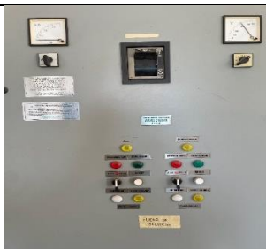
Figura 66. Interruptor principal del CCM.
