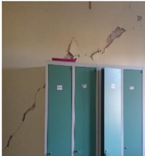
Figura 17. Falla fuera del plano. Obtenido de: Seismic performance of non-structural elements during the 2016. Central Italy earthquake
