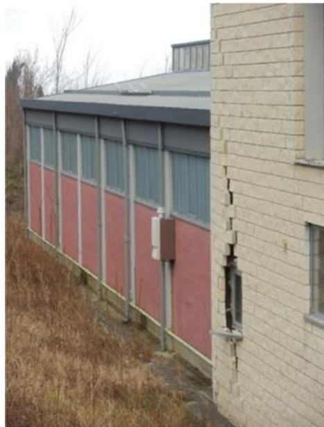
Figura 18. Falla fuera del plano Obtenido de: Seismic performance of non-structural elements during the 2016. Central Italy earthquake
