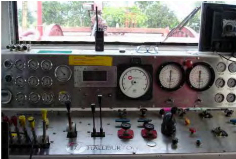
Fig. 2.6. Panel de control
