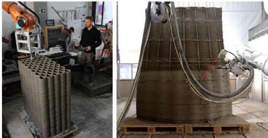
Figure 4.17: Additive manufacturing by extrusion of lightweight concrete and reinforced double-curved wall element, manufactured in shotcrete 3D printing process. Source: (Kloft et al., 2021)
