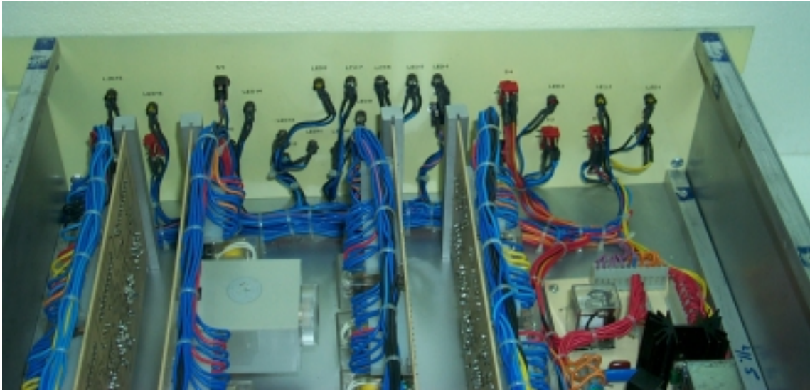
Fig. 4.15 VISTA INTERIOR DEL PANEL FRONTAL
