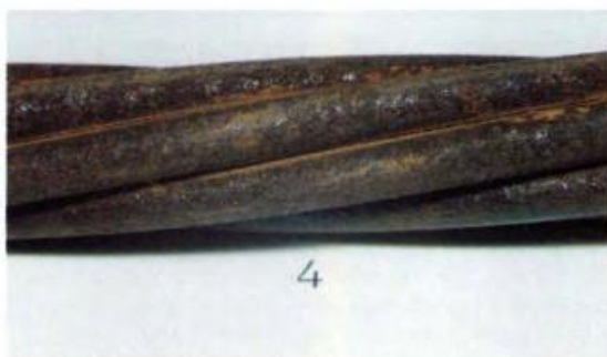
Photo 4. Strand surface before cleaning.
