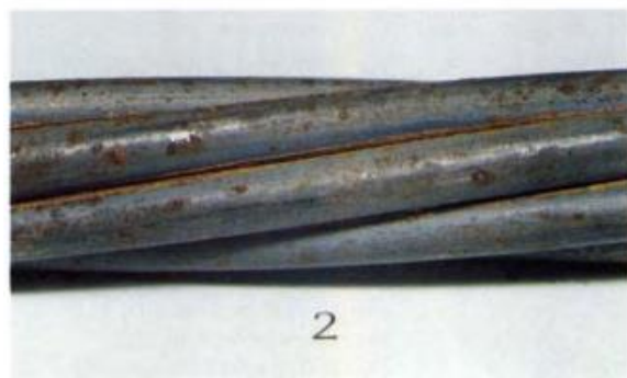
Photo 2. Strand surface before cleaning.
