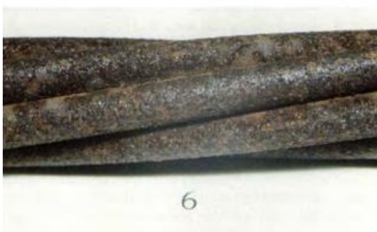
Photo 6. Strand surface before cleaning.
