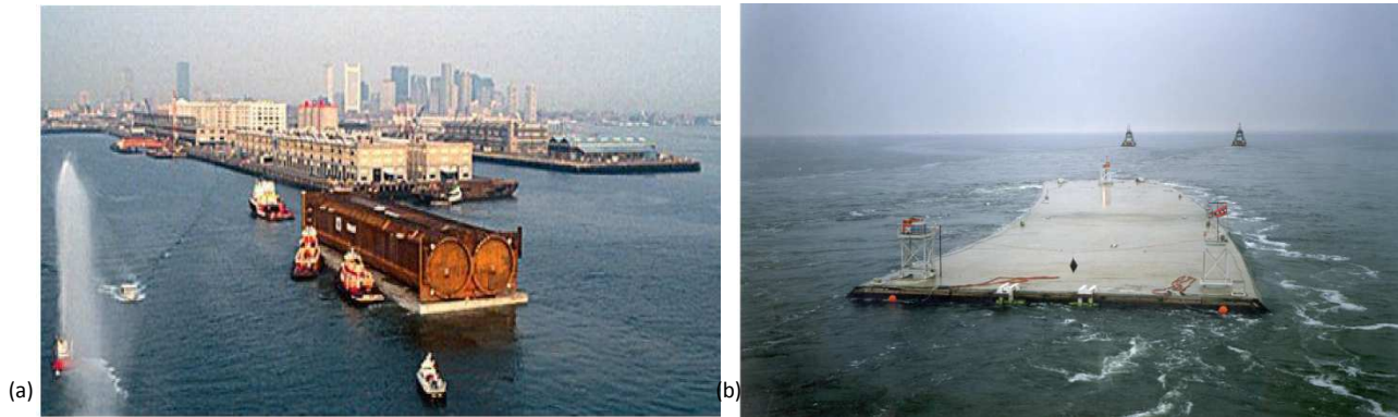
Figure 2.30 Towing process of Immersed Tunnel element: (a) Steel element; (b) Concrete element (De Wit et al., 2012)
