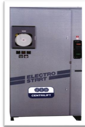
Figura 2.2 Tablero de control, Baker Hughes Centrilift Sumersible Pump Handbook, 2009.
