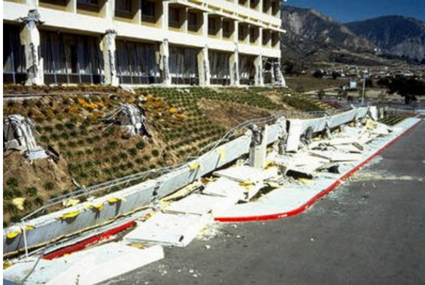
Fig 2.2 Vista del Hospital Olive View mostrando el colapso del primer nivel (The Earthquake Engineering Online Archive©)
