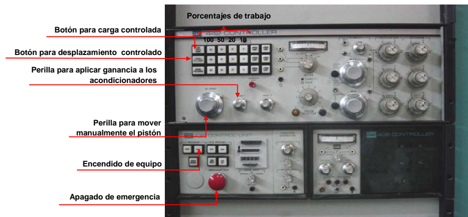
Figura 2.5 Tablero de control
