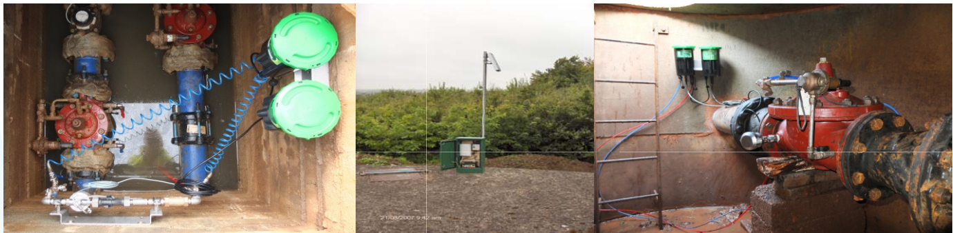
XiLogEco powered by Cla-Val (left and right) and Solar power install in Ireland (centre)
